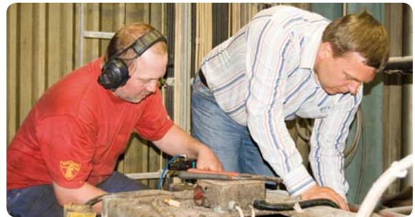
An absorbed mechanic from Bäckhammar's mill installs HISS equipment on a sootblower with Mikael Niklasson
